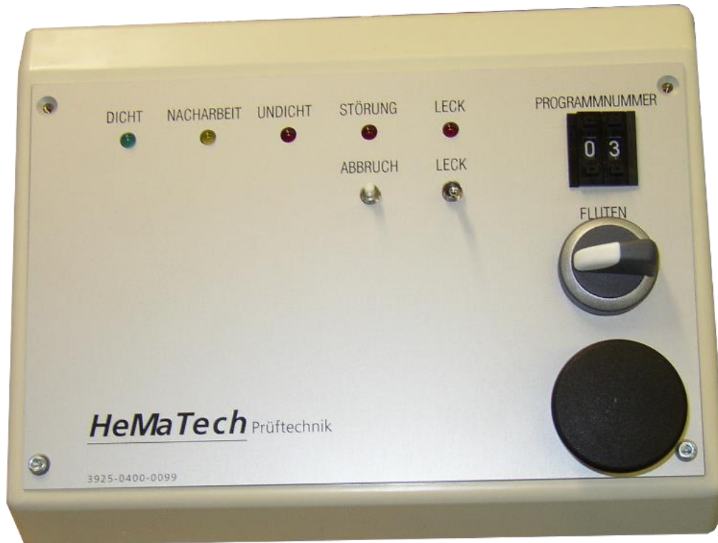
Figure 87: Manual control panel
